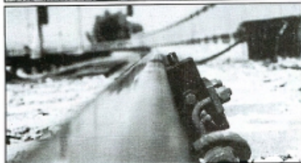
Fig. 4: Wayside lubricator installation (top), and close-up of attachment to the rail (bottom)
